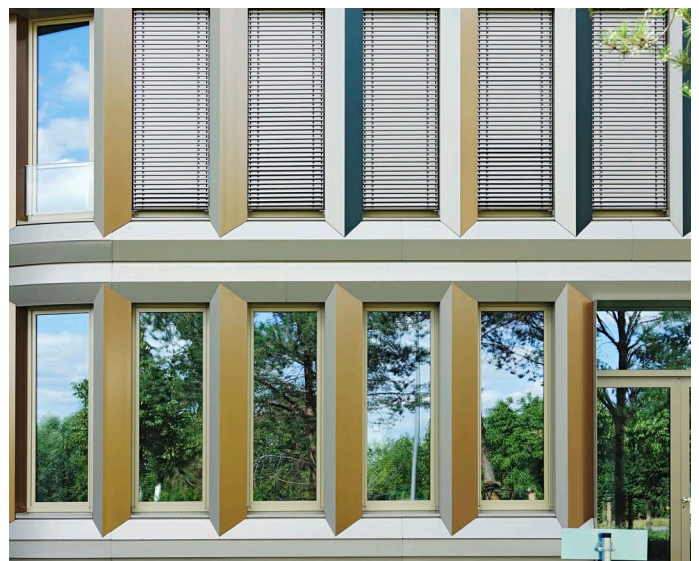
When lowered, external blinds can protect against collisions. However, this is user-dependent and therefore not suitable as a permanent solution.
