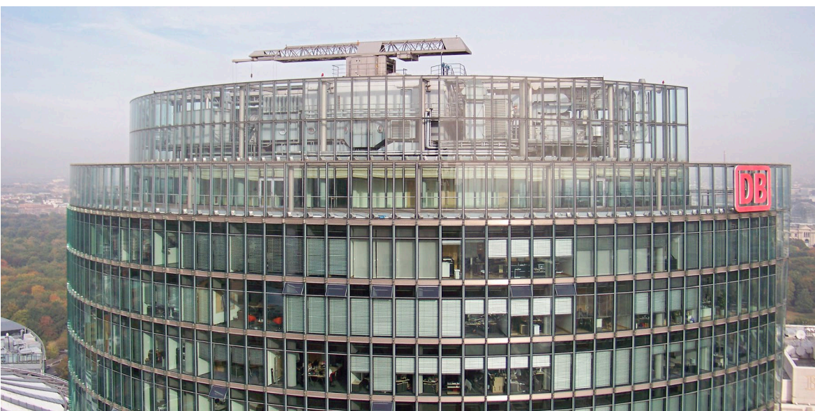
Glass parapet several metres high at the top of a skyscraper. Birds not only collide with the glass from the outside, but also hit the panes from the inside after ending up within the enclosed area.
